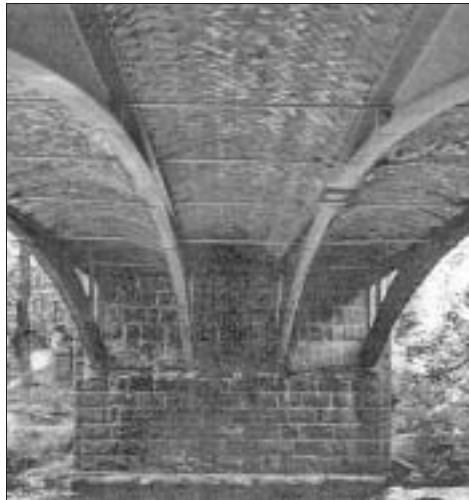
Bridge of Newe – original beams and jack-arches [Grampian Regional Council Roads Dept]
