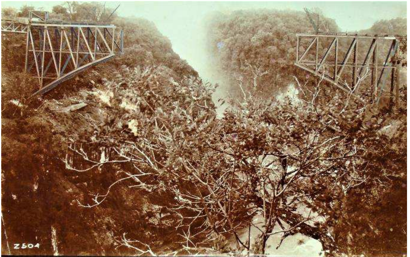
16. Victoria Falls Bridge. Albumen print. Undated c.1904?. Works progress view when arch about half complete. 8"x 6". Firm's stamp on verso. Gorge side highlighted by mist.
