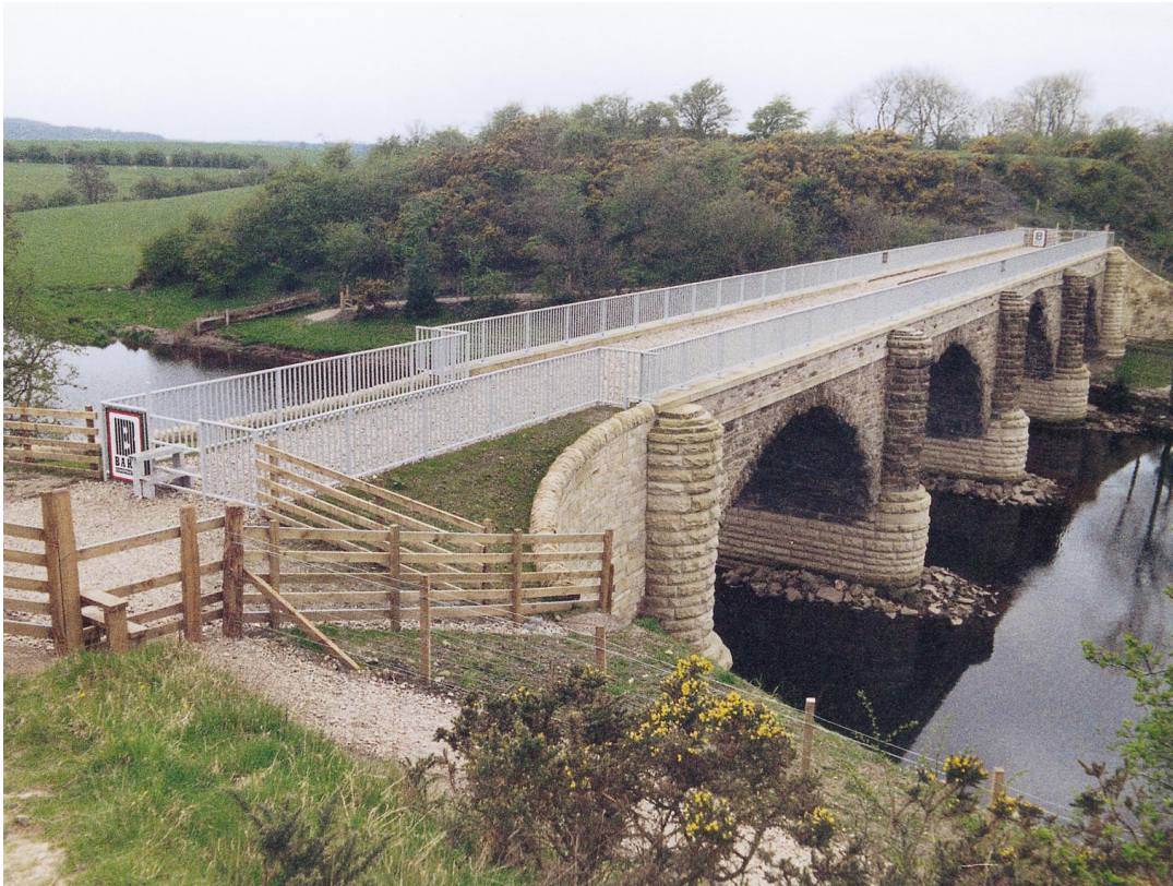
Fig. 22. North face with footpath ramps at each side, fencing and deck finishings
