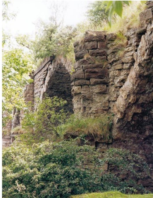
Fig. 8. West end, north face with bulging, stone loss and vegetation
