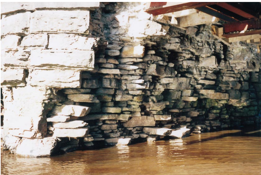
Fig. 11. West pier, east side—erosion into lime-mortar-bedded hearting (courtesy Mr F. M. Jones)
