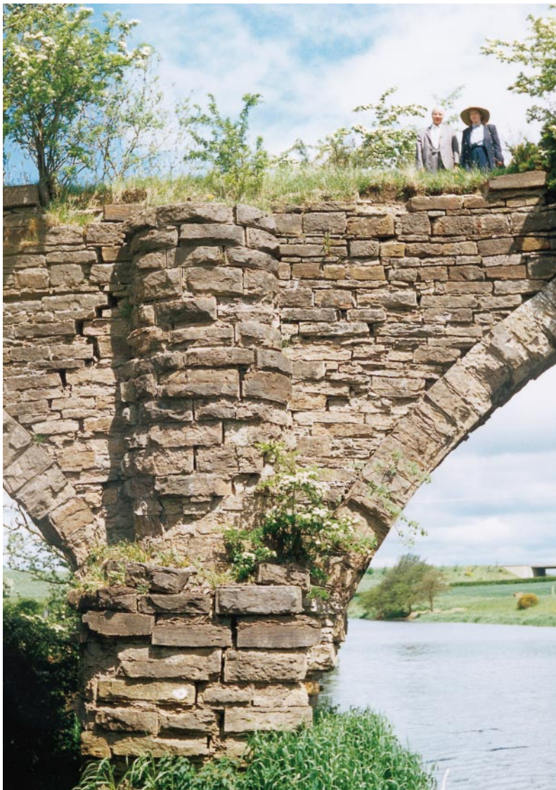
Fig. 9. (below). West pier, south face with cracking and stone loss
