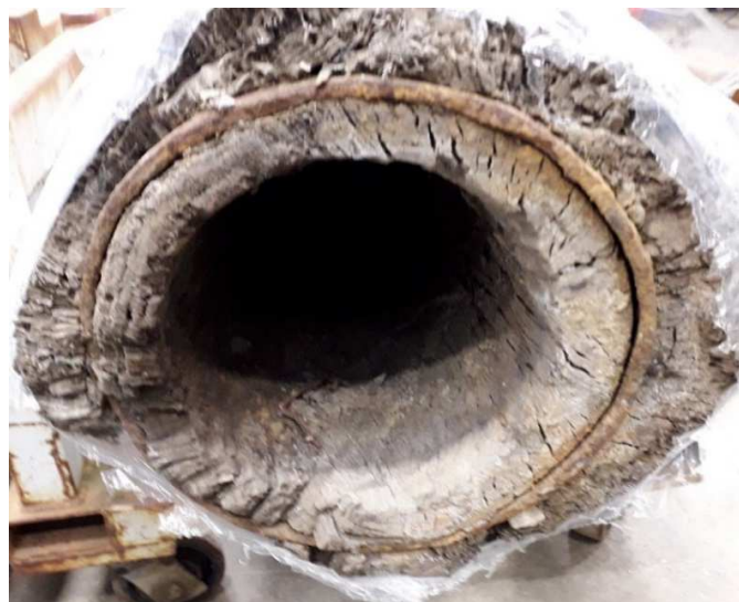
George Square pipe, iron ring in joint ©Sandra Purves
