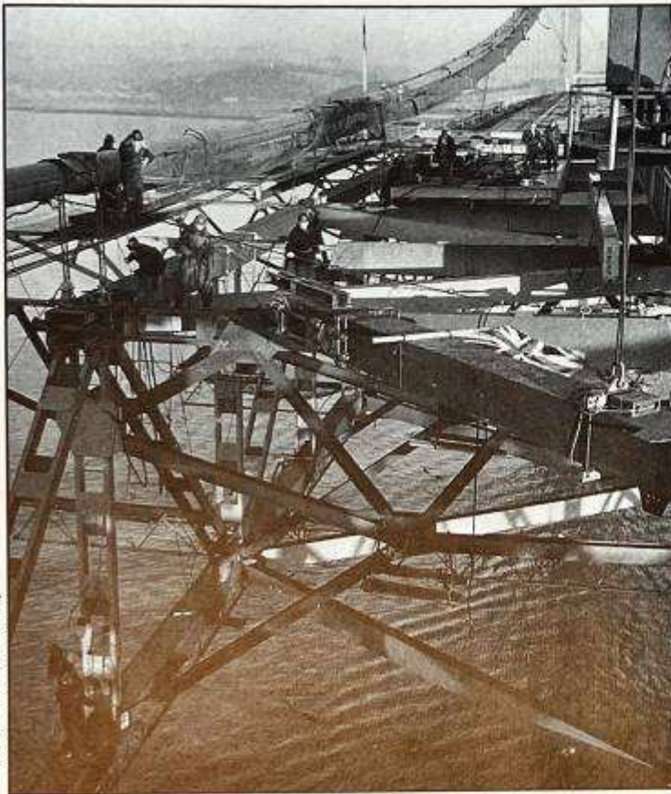
Engineers carry out the closing of the central gap, joining the north and south sections of the bridge.
