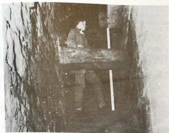
Fig. 4 — Dean Bridge. Workman standing inside the hollow spandrel on the extrados of a 96 ft span asciticuous arch. Note the stone cross-tie and the good quality of the internal masonry work. The cavities interconnected transversely by means of access holes.
