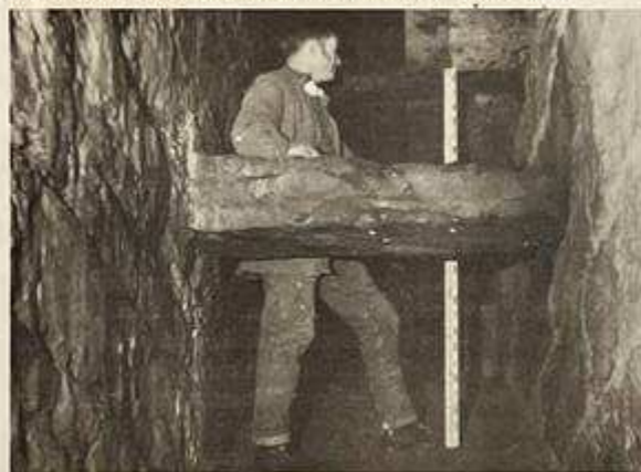
Dean Bridge. Note the stone cross-tie and the good quality of the masonry work. Telford's hollow form of construction has not only proved strong but also has greatly facilitated inspection through the years.
