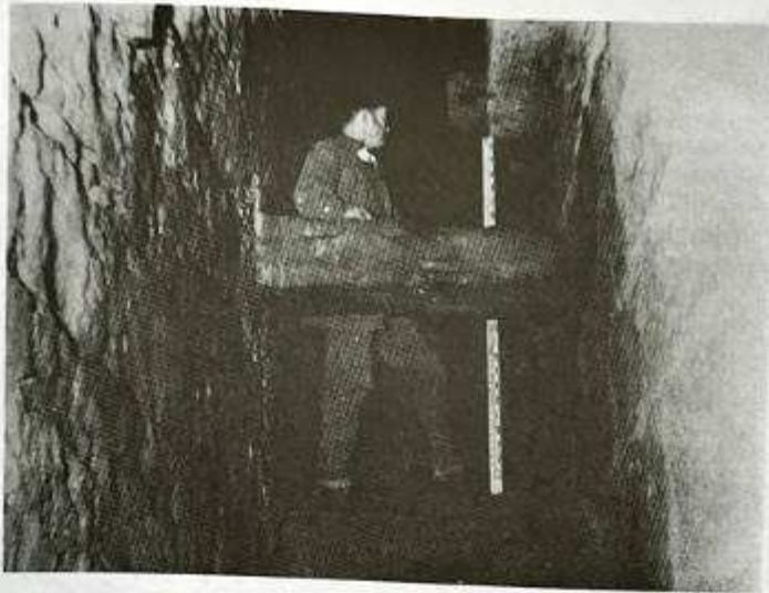
Dean Bridge. Workman standing inside the hollow spandrel on the extrados of a 96 ft span arch. Note the stone cross-tie and the good quality of the internal masonry work. The cavities are interconnected transversely by means of access holes.
