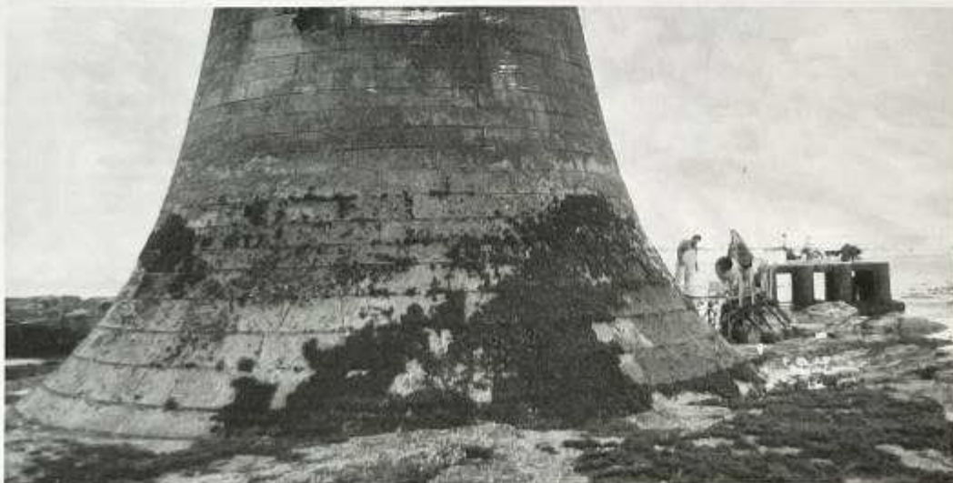
Rennie's cycloidal curves as implemented to the 42ft diameter base, checked by the editor and Robert Mackay NLB Civil Engineer when the helicopter pad was being constructed in 1986.
