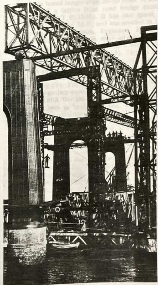
Fig. 38. Tay Bridge, Dundee under construction c.1883 — girders being transferred from the 1878 bridge for in situ strengthening and reuse
