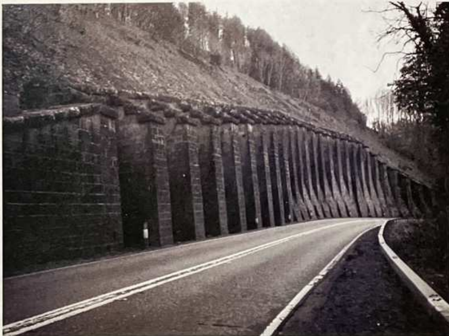
Enterkinfoot Retaining Wall supporting railway above (near tree line). R. Nith below barrier.
