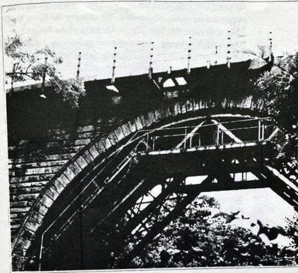
Fig. 6. Detail of the bridge prior to restoration showing the good condition of the masonry. The steel frame erected in 1968 to support the arch against possible effects of mining subsidence, and also the cantilevered footways, were removed as part of the restoration. The railway was closed to passenger traffic in 1969.
