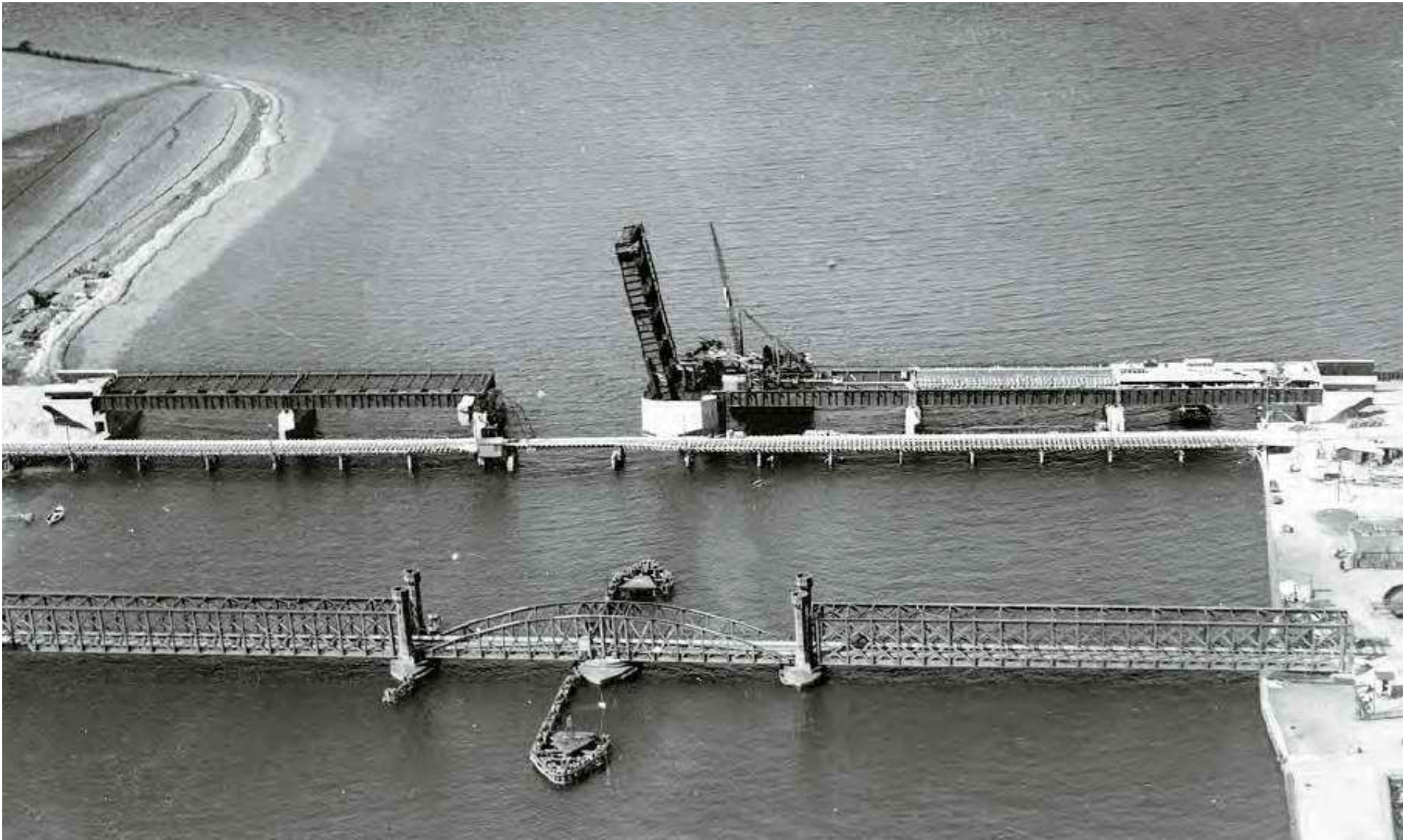
Masnedesund [road/rail] Bridge (top) connecting Falster and Zeeland, Denmark, under construction in 1934 a few months after Hunter's death [RCAHMS Guide 2000, pl. 53]
