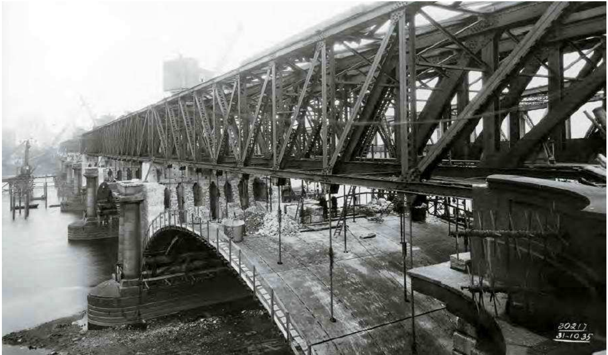
Waterloo Bridge, London, under demolition in 1935. Note Rennie's hollow spandrels of c.1813-16 to reduce weight and permit internal inspection, but some foundations eventually proved inadequate [RCAHMS 2000, pl.35]
