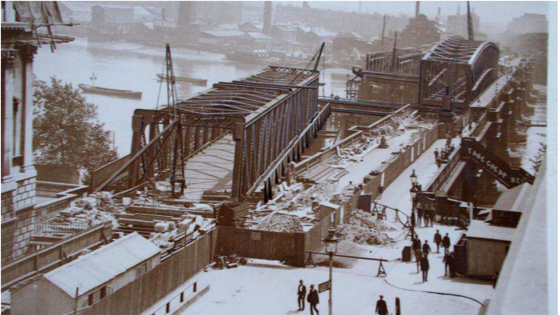
Waterloo Temporary Bridge 1924 - Rolling 280 ft long 600-ton navigation span girder into position. Temporary works design and erection under Hunter's direction [Hunter Archive]
