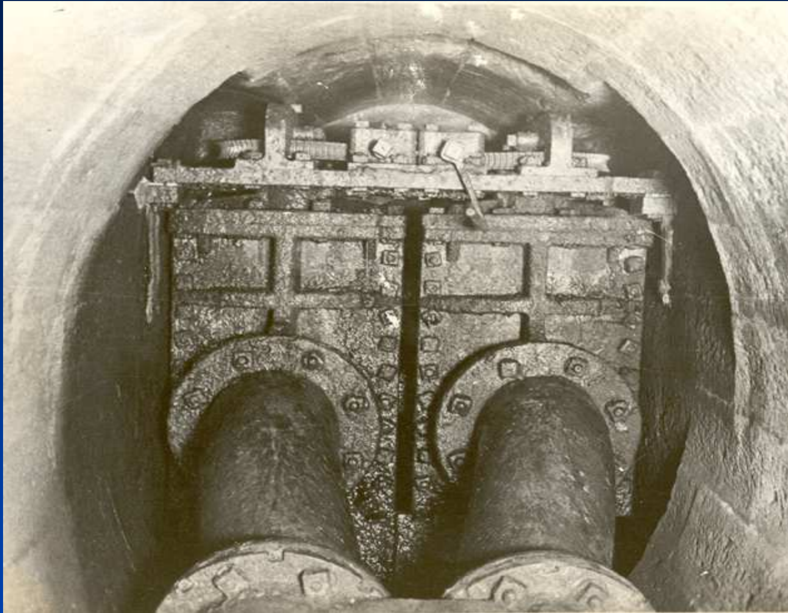
Edinburgh Water – Glencorse Dam Valves 1823
