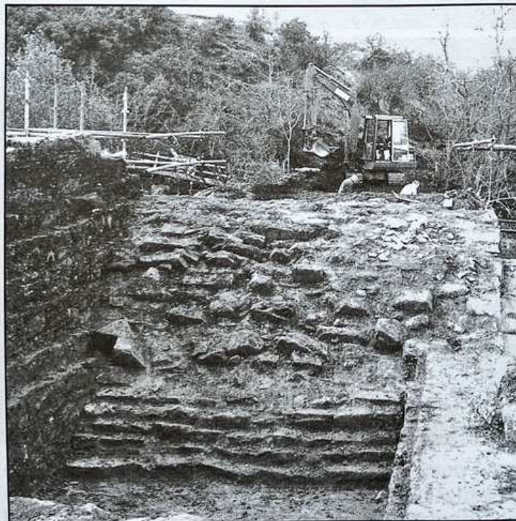
Fig 18 (top). West pier, east side — erosion into lime-mortar-bedded hearting
