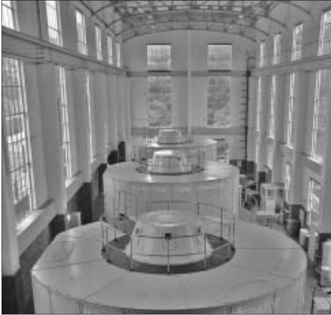
Tongland Power Station – turbo-alternator hall
