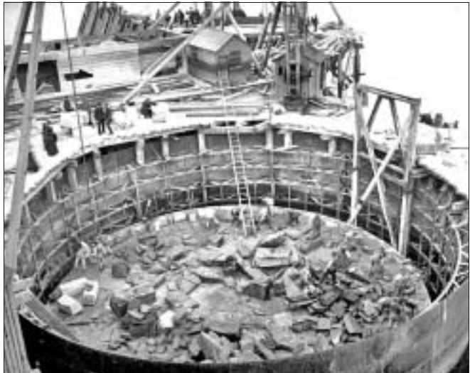
Forth Bridge – Queensferry cantilever south- east foundation under construction in 70 ft diameter caisson [photograph July 1885]
