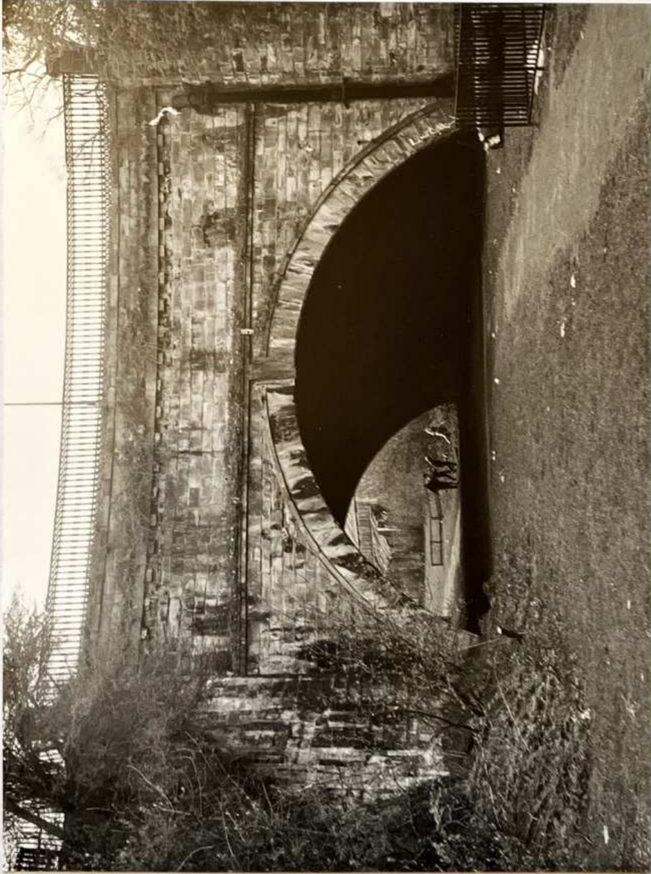
Fig 10. Luggie Aqueduct today - showing railing above former railway twin culvert entrance at right.
