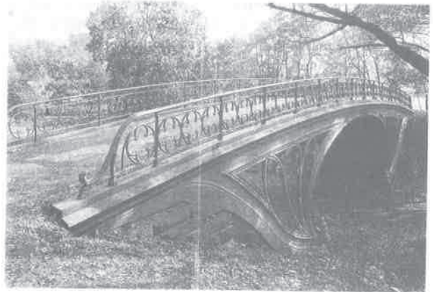
Cast-iron bridge 1861 in Central Park, New York - one of the earliest cast iron arches in the USA Courtesy of HAER and Jet Lowe
