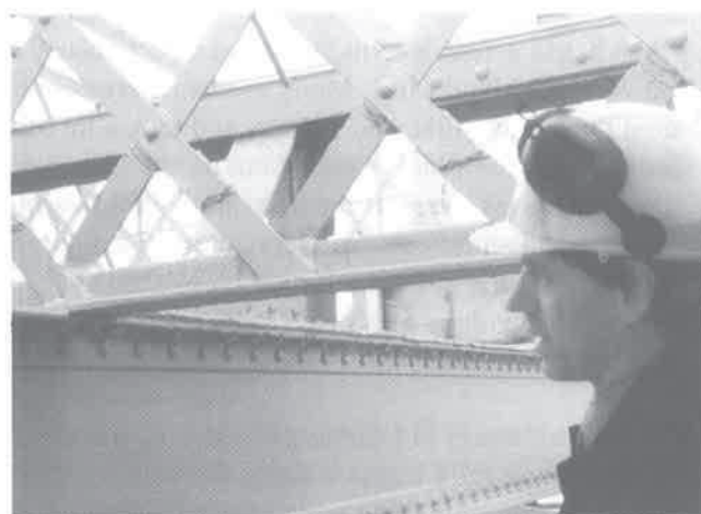
Bilston Glen Viaduct. Alan Heatley of Blyth & Blyth pointing out repairs to corroded lattice parapet on cross beam
