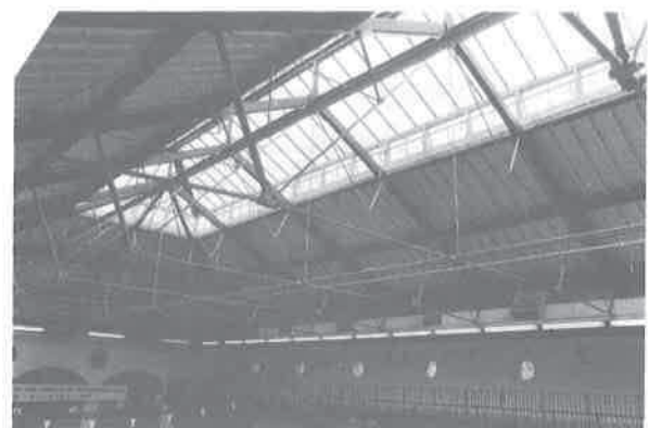
Leamington Spa Swimming Pool Roof (HEW 1742) (detail of main trusses – type M) Author's photograph
