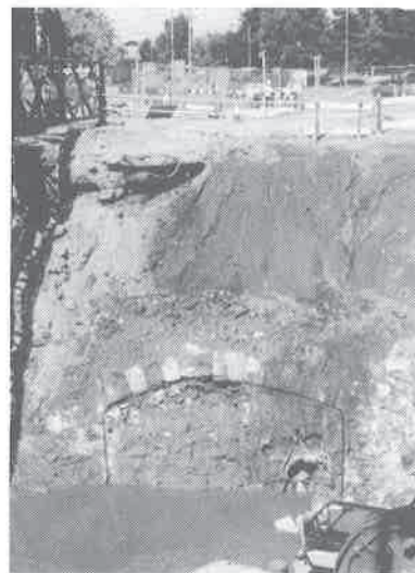
Camelon Underpass, c.1770 as seen in new lock excavation, July 2000 Photograph by Professor Paxton
