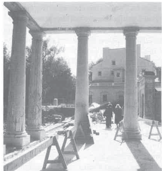
View from central pavilion (1872) towards engine house. Note condition of columns prior to restoration and the skilfully repaired timber portal on right
