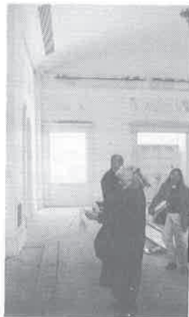
Renovated engine house showing north flywheel pit (covered). Claire Donato, architect, on right © The Author
