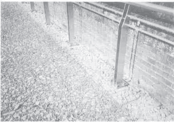
3 rd Usui Viaduct deck with surfacing and stainless steel safety rail © Dr Onoda
