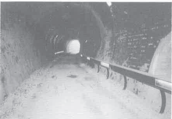
Tunnel interior – lighting fixtures, track and stone-filled side drains © Dr Onoda
