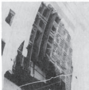
Fairmount Waterworks – roof details of 1812–1815 engine house revealed by fire damage [compare with view in Newsletter No.88] © Roland Paxton
