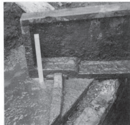
Braid Burn Bridge – Bank seat plate lug fixing detail – Effective, and probably the only surviving example © The City of Edinburgh Council
