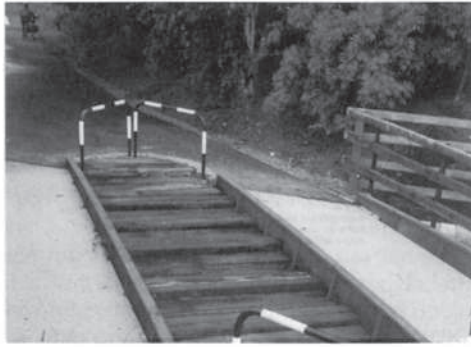
Braid Burn Bridge after being raised 0.9m – September 2001 © The City of Edinburgh Council
