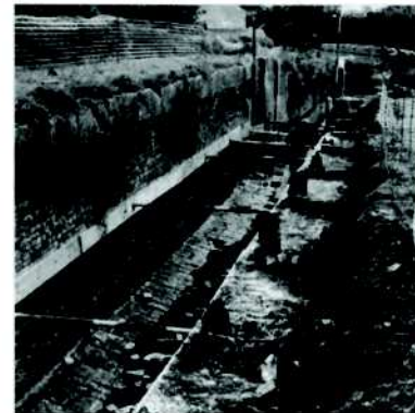
Chesterfield Canal, Turnerwood. Work being done by British Waterways' Contractors on the Thorpe Flight bottom double staircase locks. This is a Listed structure at map ref SK58SW. The timber framework can clearly be seen, also the chamber floor, and original lower brickwork, 23 September 1996.
