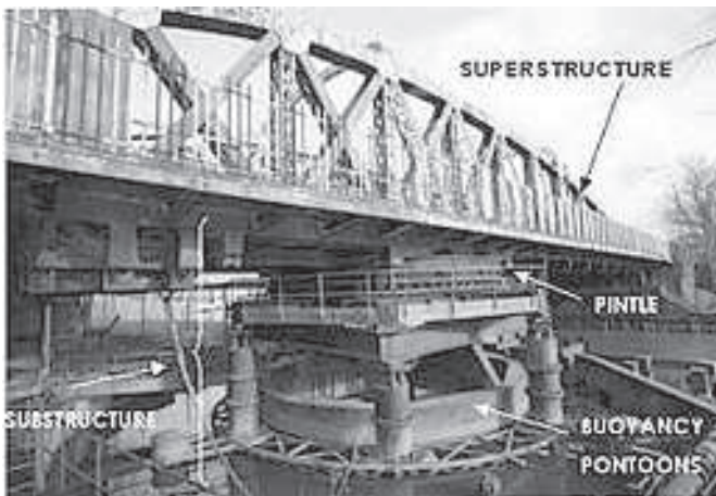
The bridge superstructure comprises a 1976 steel longitudinal trough battle deck on the central pintle span and longer nose span supported by 2004 welded mild steel girder transverse beams hung at each end from the twin
