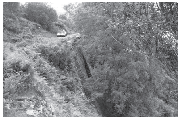
Glenelg Road ferry approach – tall retaining wall partly collapsed (1818) © R Paxton
