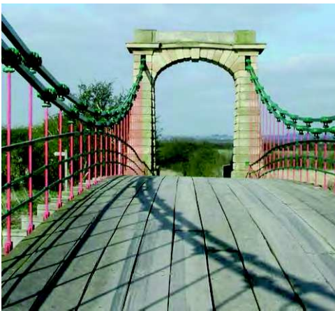
Fig. 2. Note the elegant stone tower with elliptical arch. Deck replaced by harder wood in original form ©Redmore
