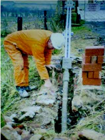
Fig. 5 Tie rod replacement of lower retained, except short corroded lengths shown ©Posford Duvivier back chain ©Posford Duvivier
