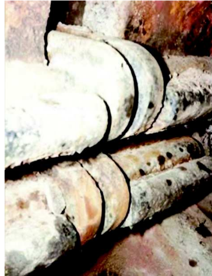
Figs 6 & 7. One of a pair of Cast Iron Anchor Plates [920x1165x100mm] in a cross-road arched tunnel [6m long x 2.2m x 0.7m wide] with its extrados at near road level. ©Redmore
