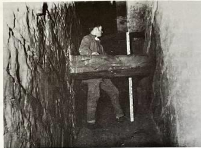
Fig. 4—Dean Bridge. Workman standing inside the hollow spandrel on the extrados of a 96 ft span asceticious arch. Note the stone cross-tie and the good quality of the internal masonry work. The cavities are interconnected transversely by means of access holes.
