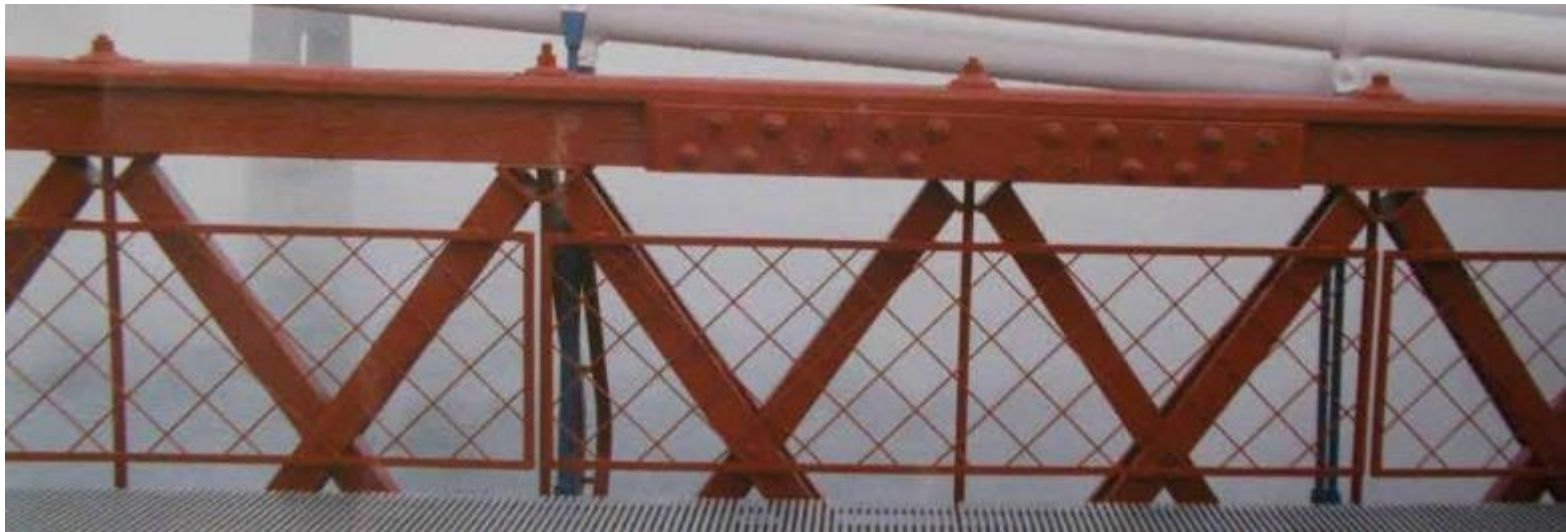
Fig. 7 - Wheeling Bridge WV USA 1849 1010ft span – Upper part of longitudinal Howe type timber trussing (rehabilitated) seen by the author in 1999. Note the adoption of wrapped, parallel multi-iron wire, main cables.
