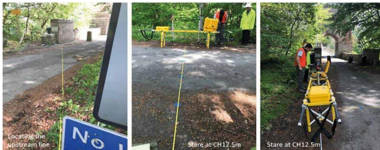
Fig. 1 [L]. Surveying line Intersections from OS benchmark location on downstream chain support wall. [M] ADR bistatic stare scan at lateral line chainage 12.5m, immediately above downstream 1820 anchor plate. View showing red Tx transmitting telescope on left of the ADR stretcher platform and the Rx receiving telescope 1 m to the right for deep focusing. [R] View of this Stare scan looking down the downstream longitudinal line with Tx sensor closest
