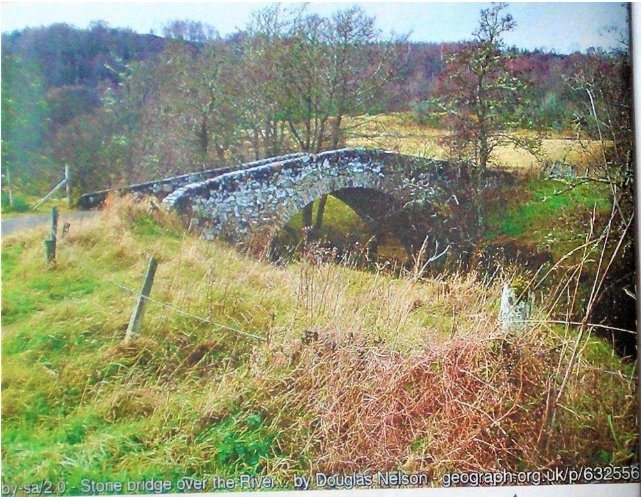
Tordarroch Bridge, 8 miles south of Inverness, is Fig. 1 Tordarroch Bridge (30ft span) Note 1 in 8 gradient on parapet tops ©Douglas Nelson
