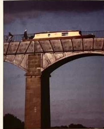
Fig. 3. Pontcysyllte Aqueduct (1805) has 19 cast-iron spans of 13.7 m and is still in use today as part of the Llangollen Canal
