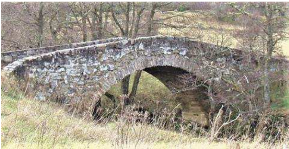
Fig. 1 Tordarroch Bridge (30ft span) Note 1 in 8 gradient on parapet tops ©Douglas Nelson
