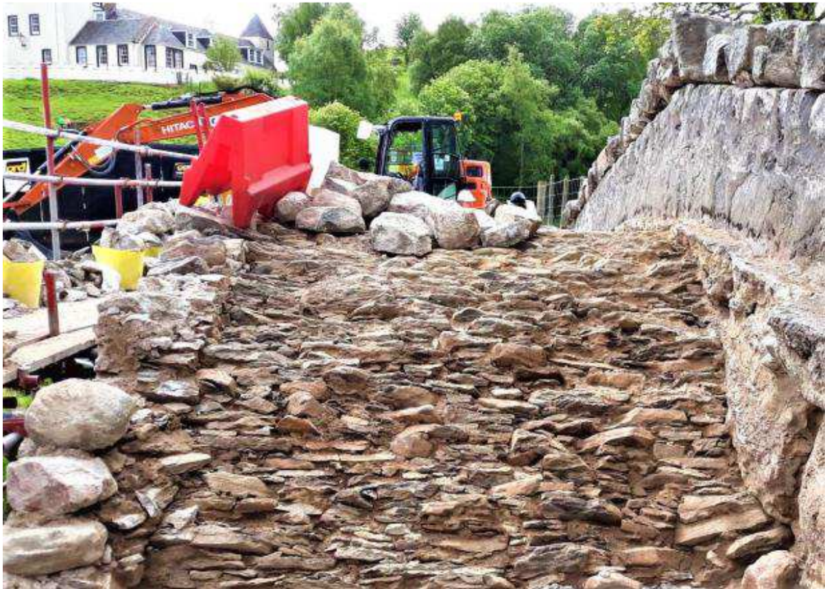
Fig. 9 Tordarroch Bridge repair in 2022 after a parapet collapse – Note the traditional, undressed, arch ring top of tightly packed thin stones under the roadway after c.240 years in service ©The Highland Council
